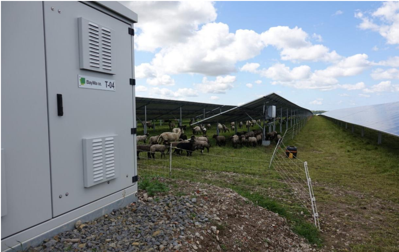
Plate 3: Typical transformer on a solar farm site
